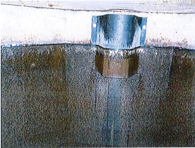
Inlet baffle of 2 nd 1500 gallon tank
