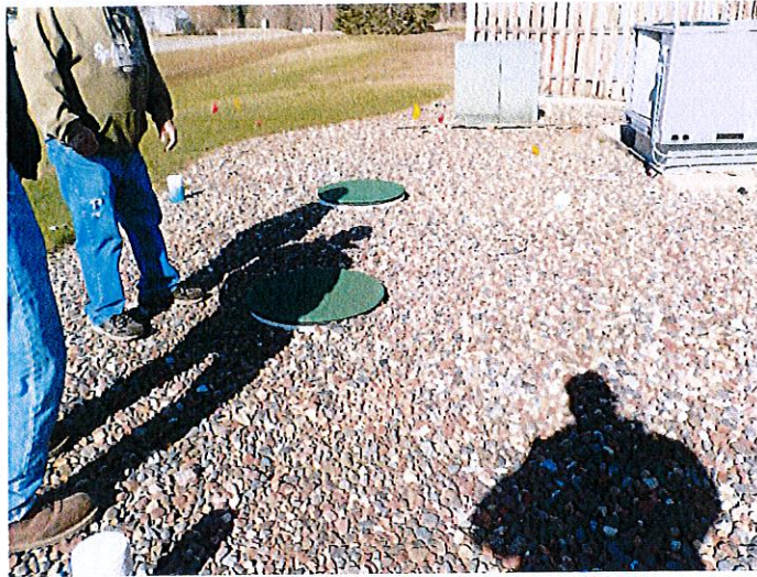
1 st tank & 2 nd tank
