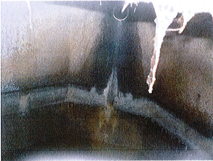
Inlet of the 1000 gallon pump tank
