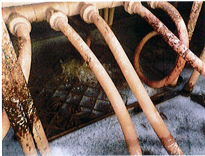
Inside of the nibbler tank
