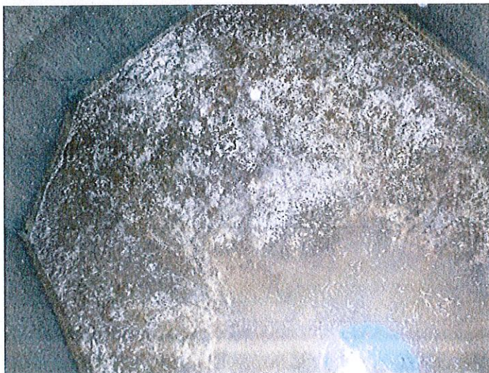
floor of the 2 nd 1500 gallon tank
