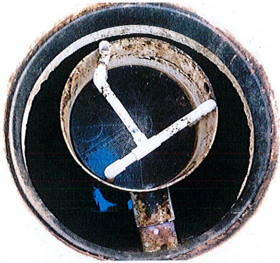
Inside of the filter chamber
