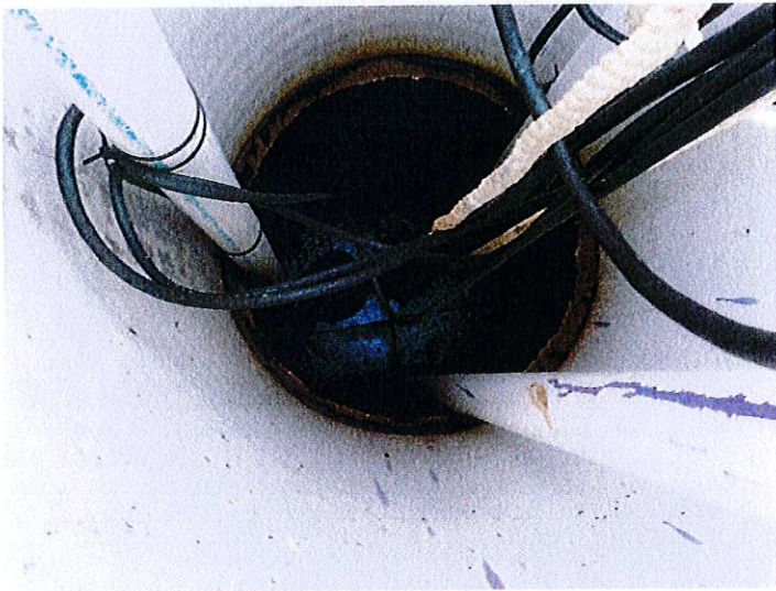
Inside of the pump tank
