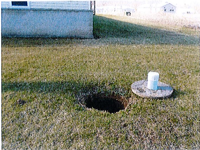
1 st 1500 gallon septic tank at office
