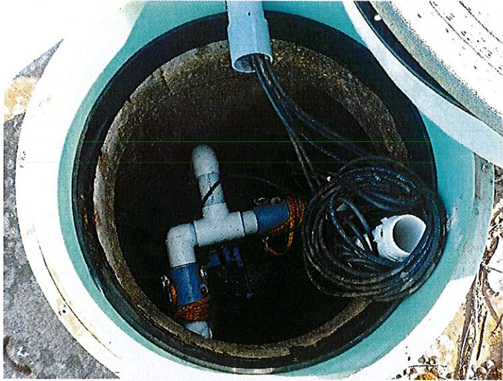
Inside the pump tank
