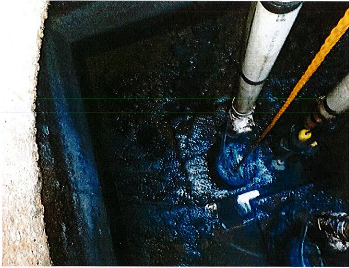
Side wall and pumps
