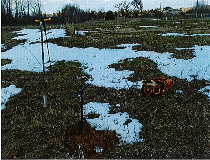
System area and soil boring 1
