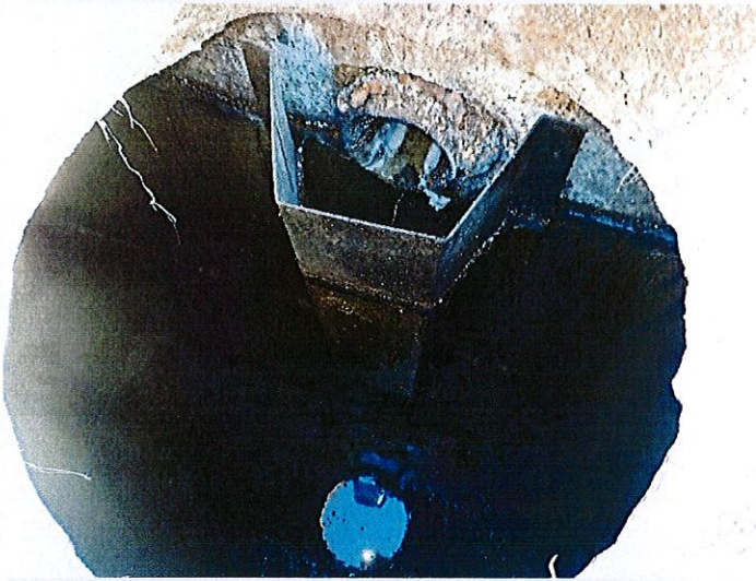
Outlet of the 1 st 6000 gallon tank
