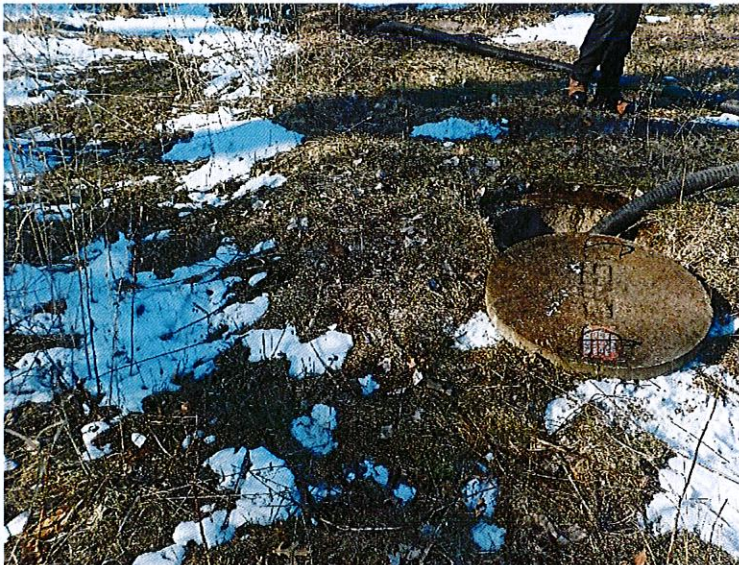
6000 gallon septic tank
