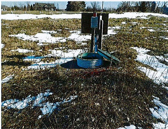
2000 gallon pump tank
