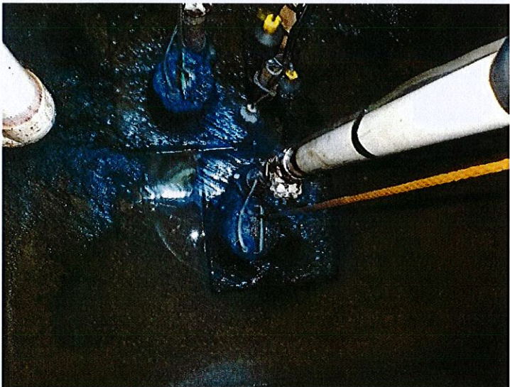
Floor and pumps
