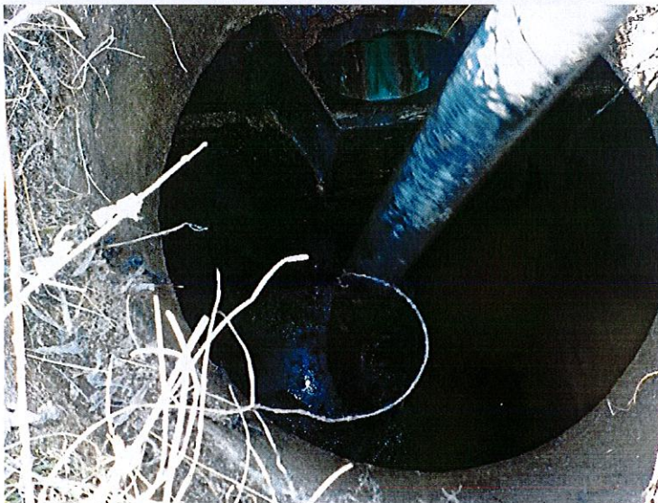
Inlet of 1 st 6000 gallon tank
