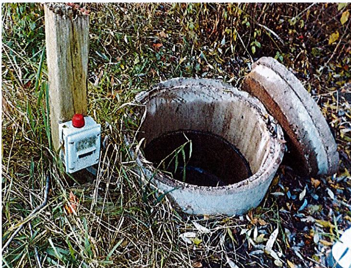
Alarm for filter
