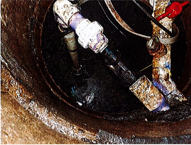
Inside pump tank
