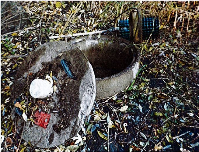
Chipped cover on filter tank
