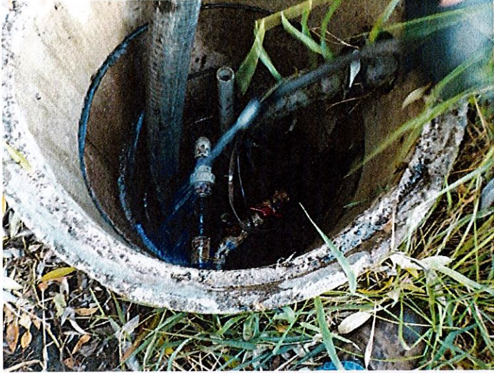
Inside pump tank
