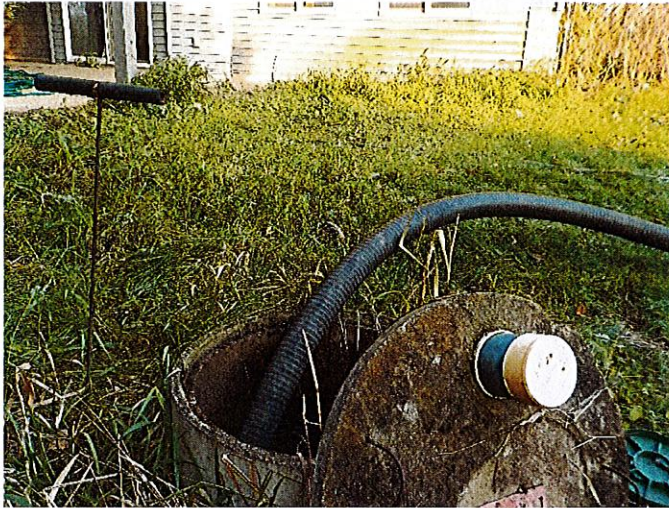
2000 gallon septic tank
