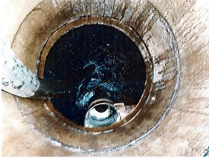
inside filter tank
