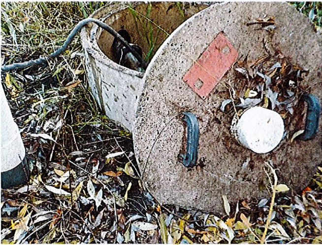
Chipped cover on pump tank
